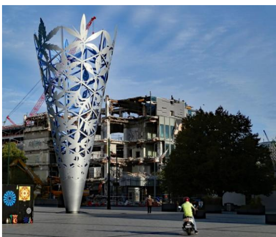
After the Earthquake
